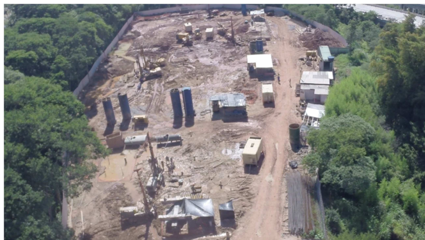
Figure 7. Project site at the beginning of the installation of the root piles
