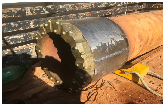
Figure 2. Last cutting tool used to install the root piles (Saez et al., 2020)
