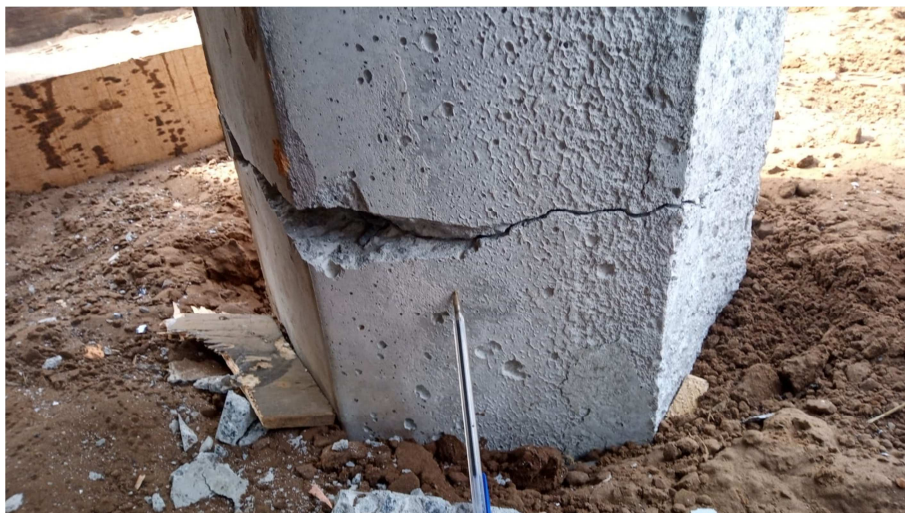
Figure 5. The damaged area of the 45cm-hexagonal pile
