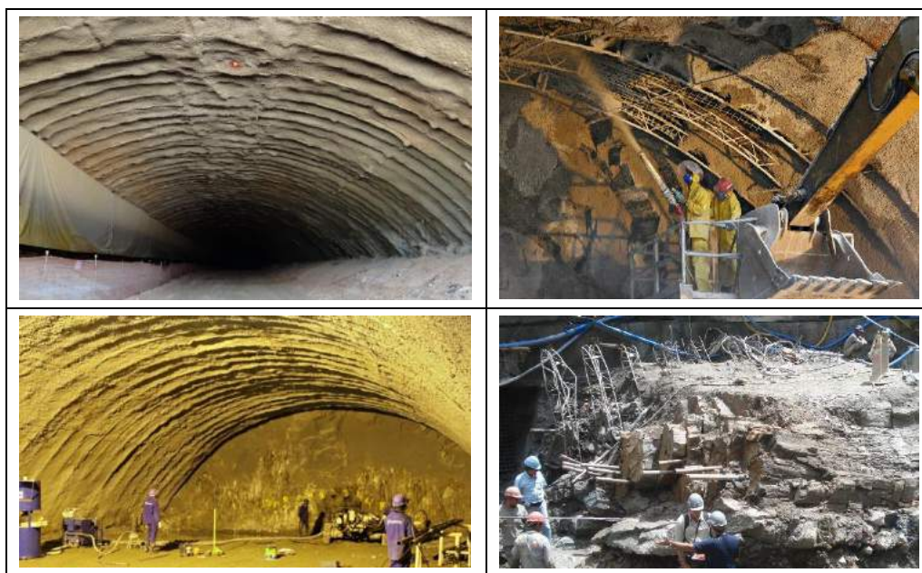
Figure 15 - The use of lattice girders in the temporary support phase of NATM has it's own special challenges when there is over-break, since shotcrete volumes needed to spray in the steel bars may be very large. These two examples (a section of motorway and a section of cavern) failed dramatically and in one case tragically, due to non-uniform loading of the lattice-girders which are too 'soft' since unbolted, therefore can bend and also need non-yielding 'elephant feet' (BARTON, 2017).
