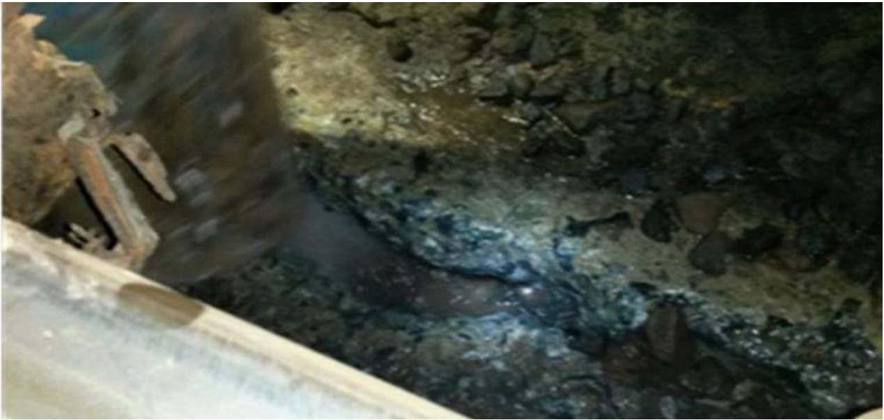
Figure 2 - Crack on the floor slab
